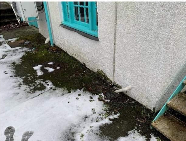
Moss growth to tarmac surface to building perimeter.
